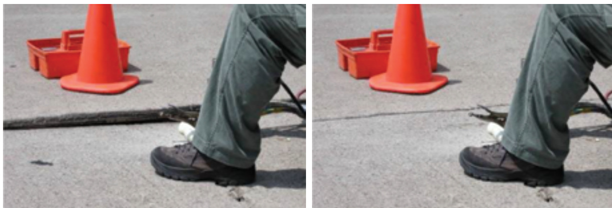
Figure 4.4. Settled slab before (left) and after (right) slab jacking (courtesy of John Roberts, International Grooving and Grinding Association [IGGA])
