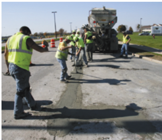
Figure 5.21. Placement of repair material for long joints using mobile concrete truck (Frentress and Harrington 2012)
