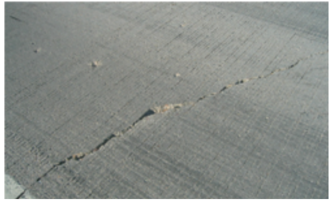
b. Transverse cracking
