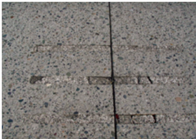
a. Cracking within dowel bar slot
