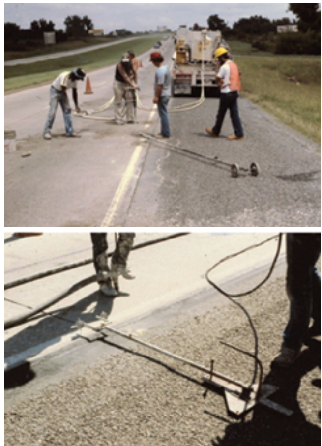
Figure 4.13. Methods of monitoring slab uplift (photos courtesy of Wouter Gulden, retired Georgia DOT)
