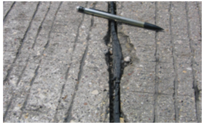
f. Joint seal damage
