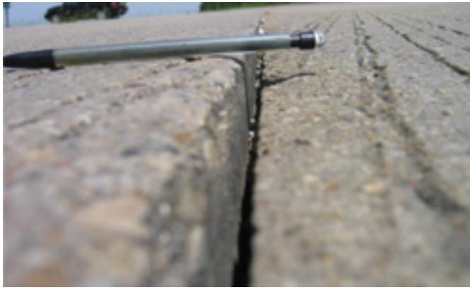
a. Joint faulting
