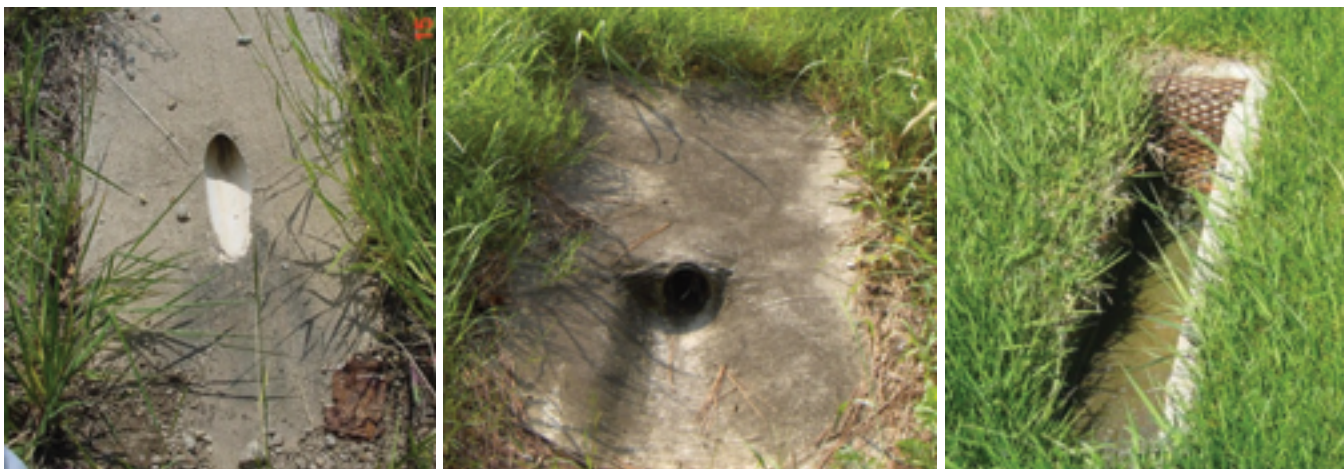
Figure 7.15. Various headwall installations
