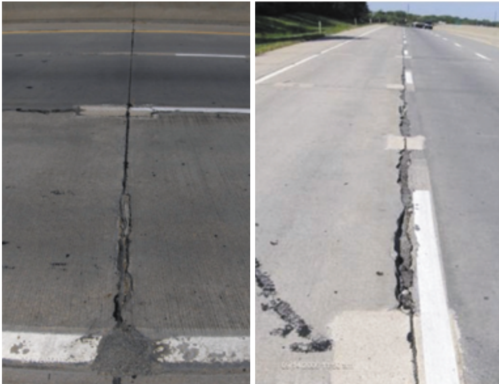
Figure 5.3. Candidates for Type 2 repairs (Frentress and Harrington 2012)
