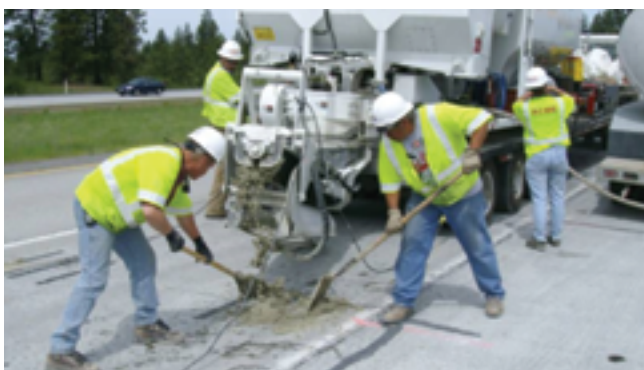
Figure 8.15. Placing patching material into the dowel bar slot (Pierce, Uhlmeier, and Weston 2009).
