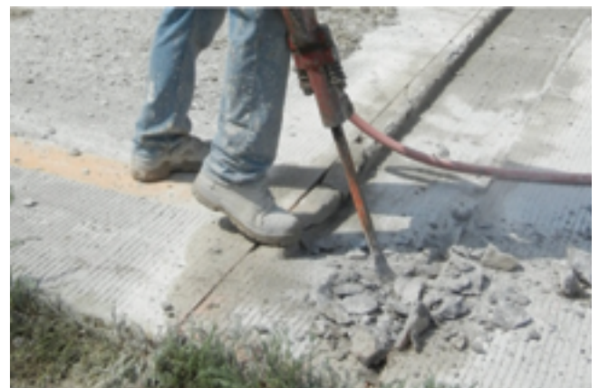
Figure 5.12. Repair area prepared using the chip-and-patch (Types 1 and 3) procedure
