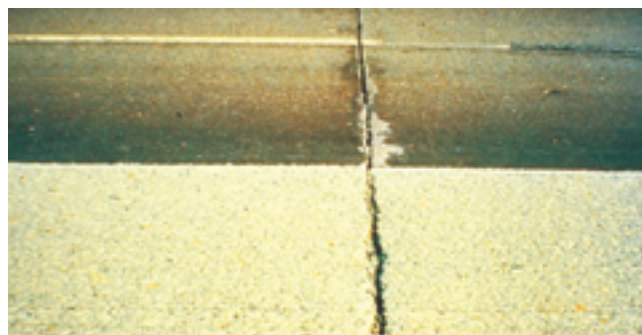
Figure 9.8. Joint damage (foreground) caused by cold milling
