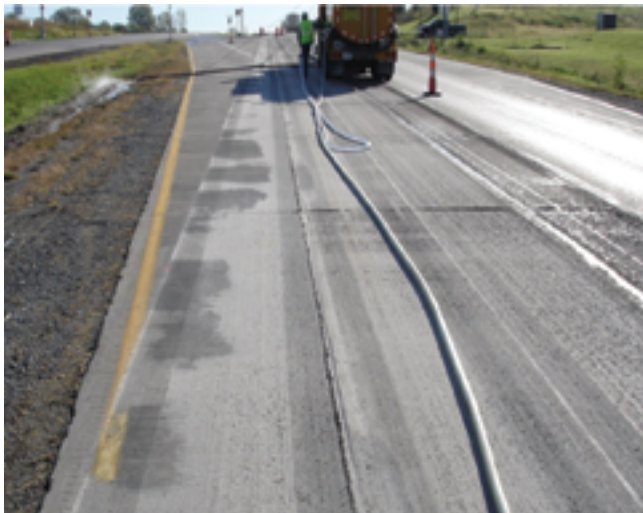
Figure 9.16. Holidays on diamond ground surface of inside turning lane (courtesy of Dan Frentress, IGGA)
