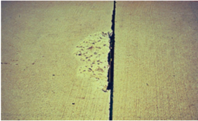
c. Joint spalling
