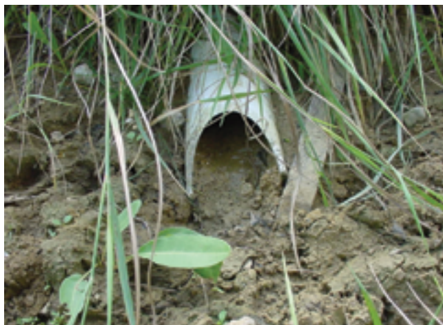
Figure 7.17. Clogged outlet pipes (courtesy of John Donahue)
