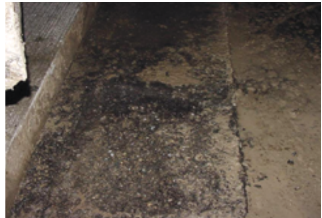
Figure 11.9. Stripping of asphalt interlayer (photo courtesy of Dan DeGraaf, Michigan Concrete Association)
