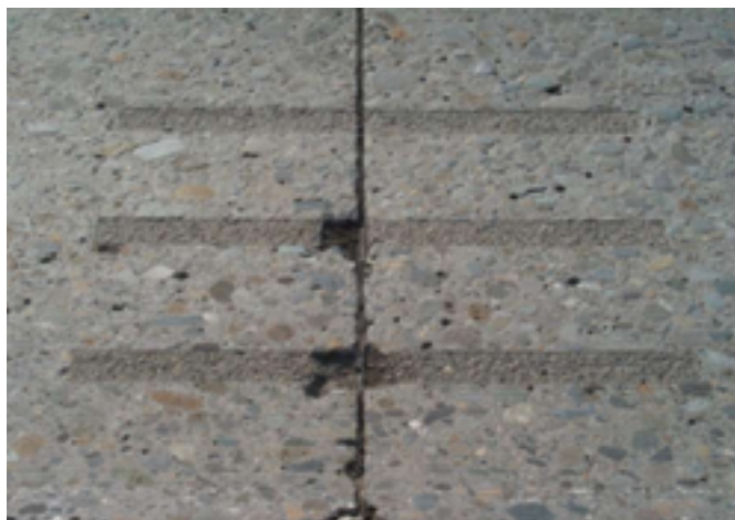
c. Spalling within dowel bar slot
