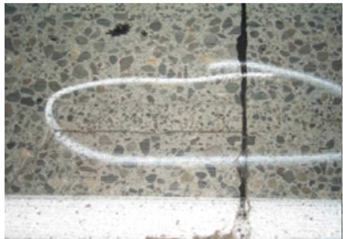
b. Debonding of patching material
