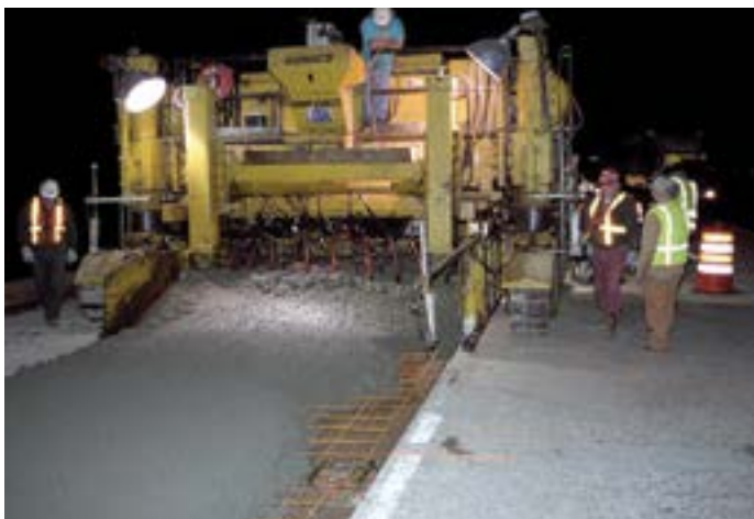
Figure 99. Controlling paving profile using a paver ski on the adjacent lane (source: Wouter Gulden, southeast chapter, ACPA)
