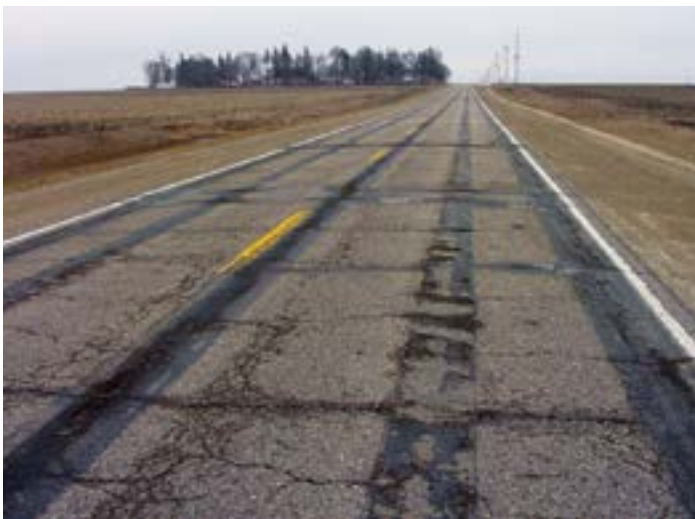
Figure 34. Poor to deteriorated asphalt pavement to be resurface (source: Todd Hanson, Iowa DOT)
