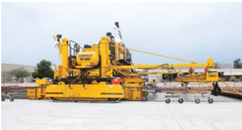
Figure 98. Controlling paving profile using a moveable stringline on the adjacent lane (source; Kevin Klein, Gomaco)
