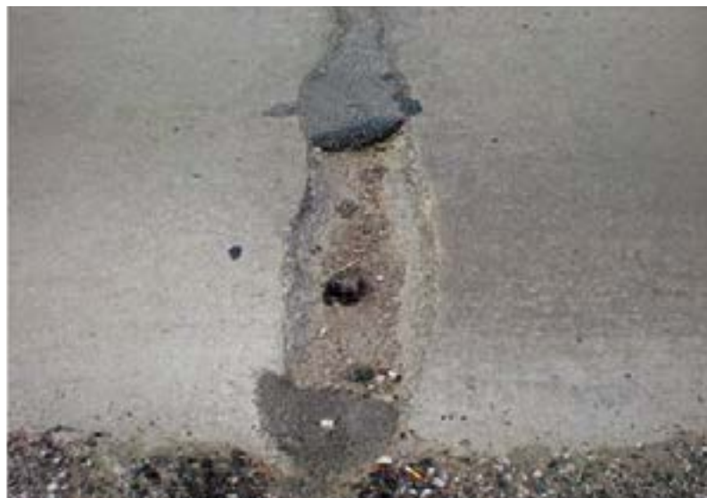
Figure 12. Typical joint deterioration with HMA patch (source: Trinity Construction Management Services, Inc.)
