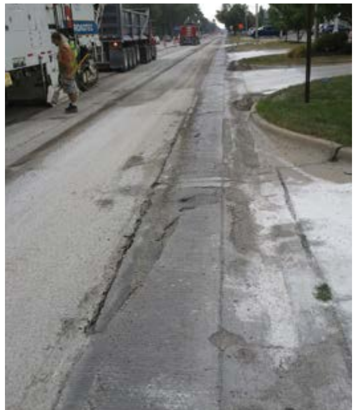
Figure 119. Typical concrete pavement milling operation (source: Dan DeGraaf, Michigan Concrete Paving Association)
