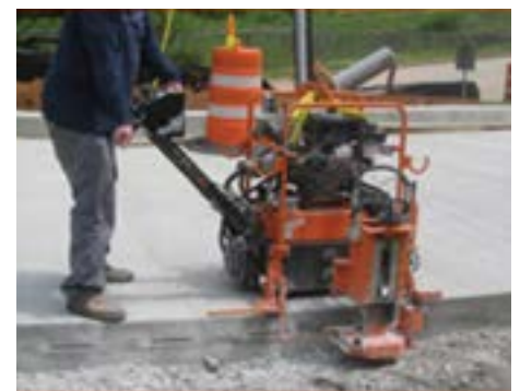
Figure 69. Slots being cut to accept the football-shaped plate dowels (source: Nigel Parks, PNA Construction Technology)
