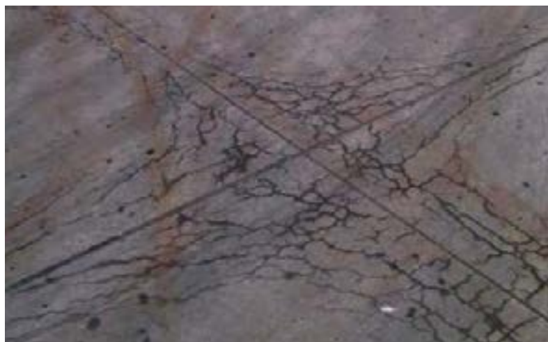
Figure 10. Moderate ASR cracking along the perimeter of slabs (source: [Thomas et al. 2011])
