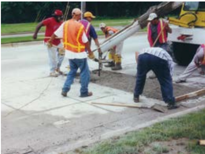
Figure 117. Finish and cure of concrete overlay repair (source: Dan DeGraaf, Michigan Concrete Paving Association)
