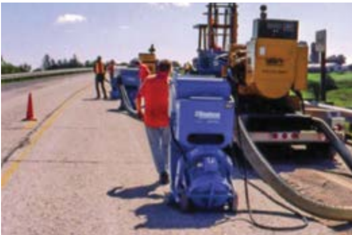
Figure 28. Photo of concrete pavement with shotblast surface prior to concrete overlay in 1994 (source: Todd Hanson, Iowa DOT)
