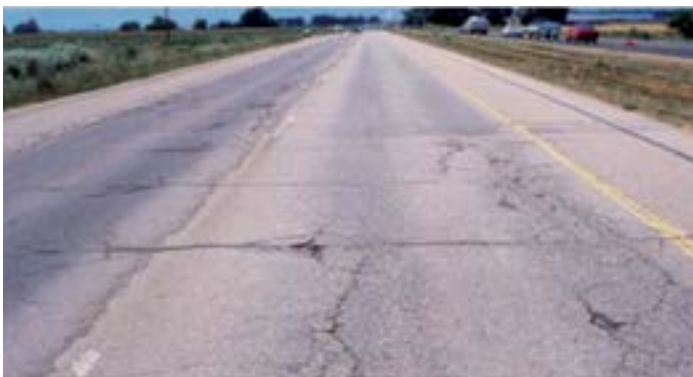
Figure 19. SH-119 in 1991 prior to placement of an bonded concrete overlay (source: Ron Youngman, CO/WY chapter, ACPA)
