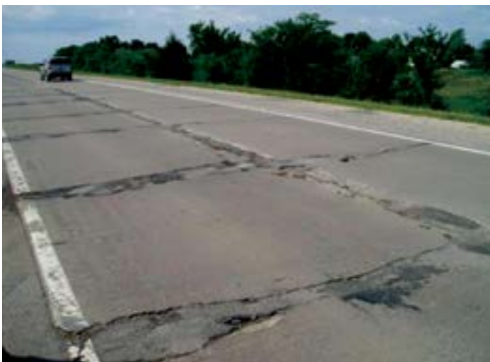
Figure 44. Route D35 existing pavement in poor condition (source: Todd LaTorella, MO/KS Chapter, ACPA)
