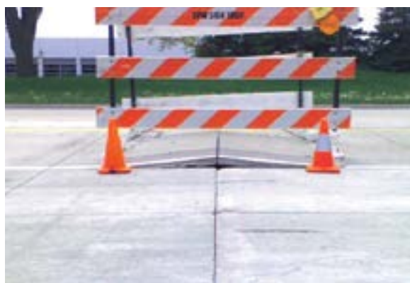
Figure 52. Overlay blowup where expansion joint should have been cut over existing concrete expansion joint (source: Dan DeGraaf, Michigan Concrete Paving Association)
