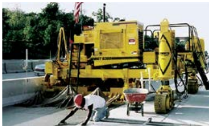
Figure 96. A three-track, zero-clearance paver placing concrete along a median barrier (source: Kevin Klein, Gomaco)
