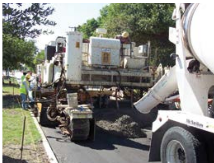
Figure 97. A typical four-track paver modified to three tracks, providing zero clearance in a C/G situation in Oklahoma (source: Jim Duit, Duit Construction Co., Inc.)
