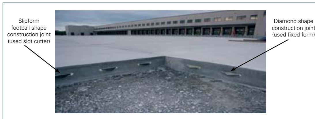
Figure 65. Diamond-shaped plate dowels in fixed-formed construction joints (right side) and football-shaped dowels by slipforms
