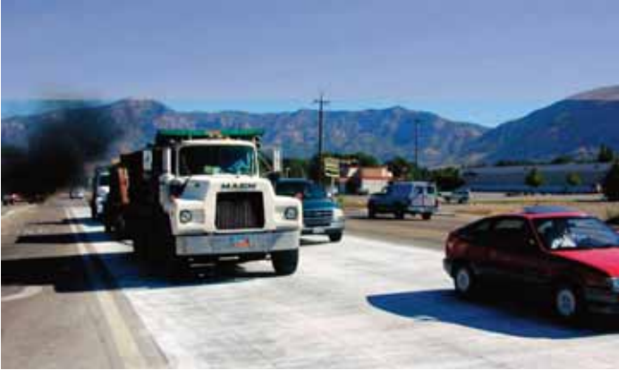
Figure 2-13. A 4-in. (100-mm) thick bonded concrete overlay on an existing asphalt pavement on a city street in Ogden, Utah.
