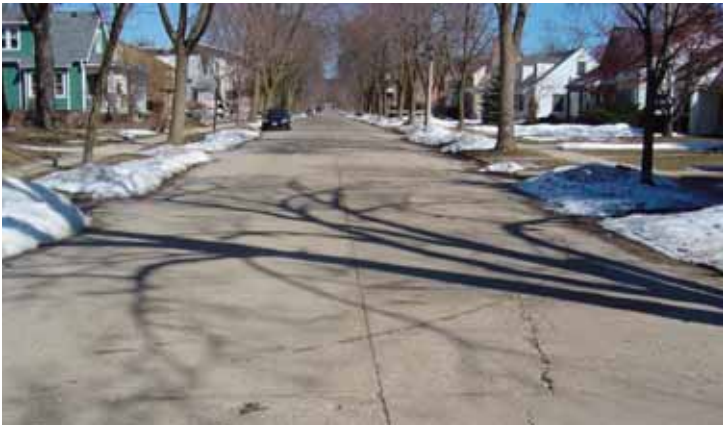
Figure 3-1. Existing 80-year-old concrete pavement.
