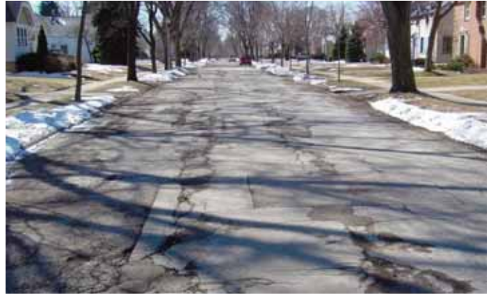
Figure 3-2. Existing 34-year-old asphalt pavement.
