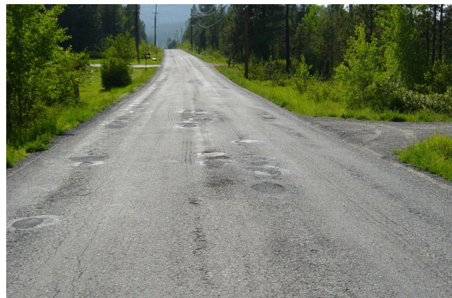
Figure 3.1. Excessive patching on asphalt roadway
