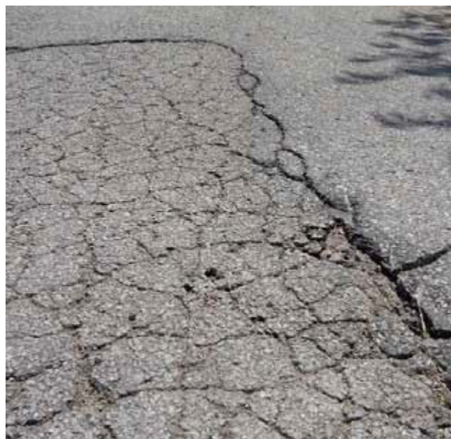
Figure 3.7. High-severity alligator cracking
