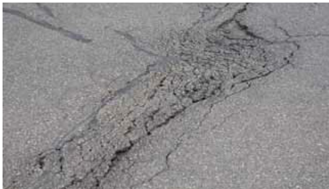
Figure 3.11. Low- to medium-severity pothole
