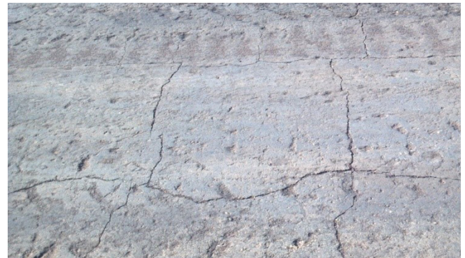
Figure 3.10. Block cracking on a compacted CTB layer
