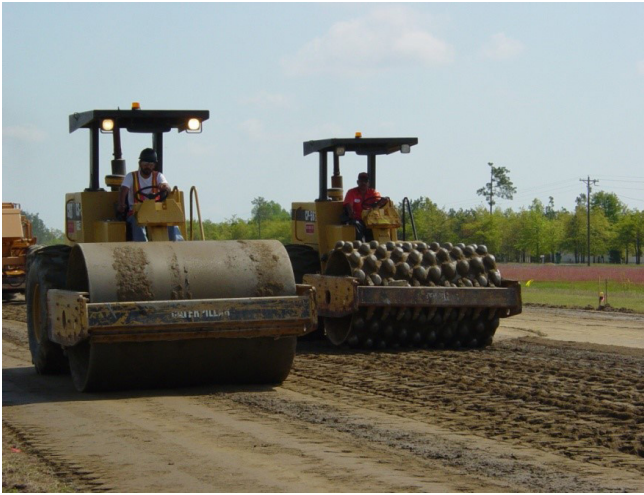
Figure 1.12. Final compaction of FDR base with a tamping roller (right) and a smooth-wheeled vibrating roller
