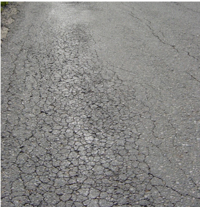
Figure 1.6. Asphalt pavement with extensive alligator cracking
