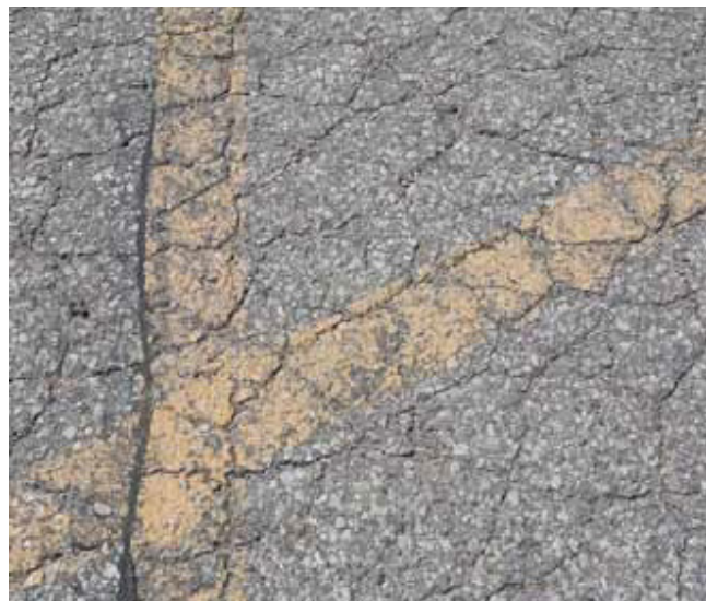
Figure 3.6. Low- to medium-severity alligator cracking
