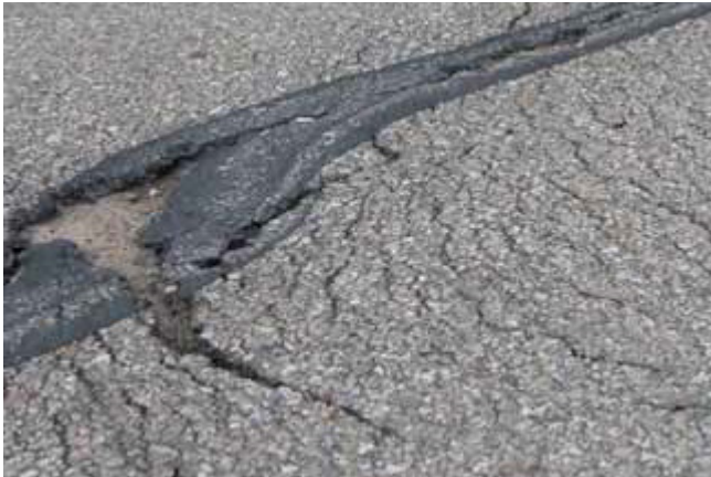
Figure 3.15. Low- to medium-severity shoving
