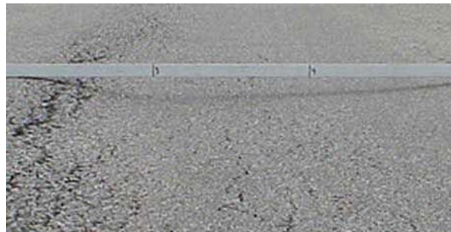
Figure 3.13. Low- to medium-severity rutting
