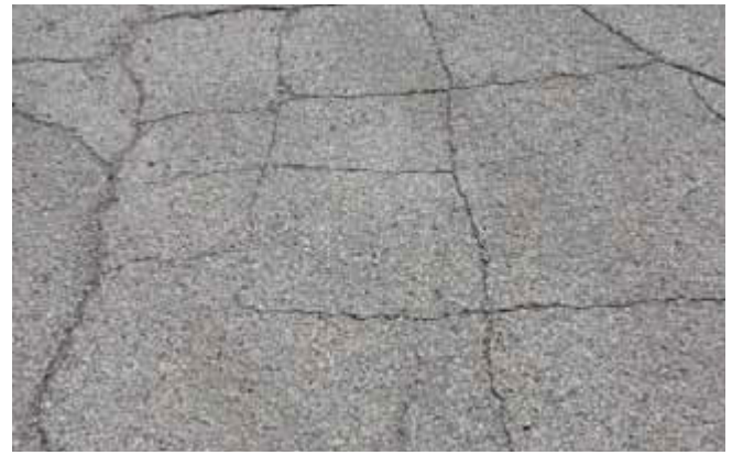
Figure 3.8. Low- to medium-severity block cracking
