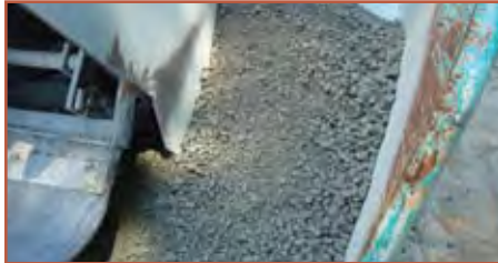
Segregation in paving hopper
