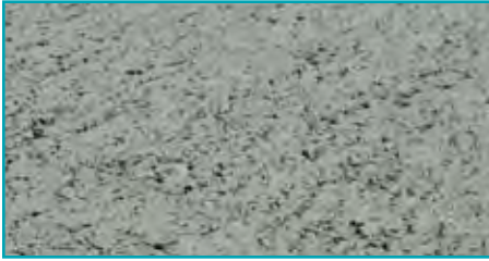
Mix too dry
