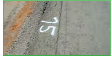
Required target density is not achieved
