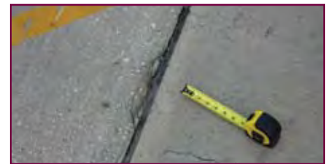
Spalling at cold joint
