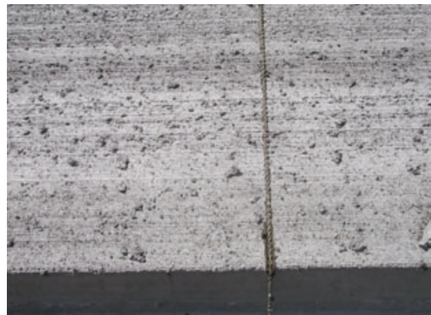
Figure 6.4. Photo of Minnesota concrete pavement textured by Astroturf drag prior to joint sawing and pavement sweeping (photo provided courtesy of Mr. Doug Schwartz, Minnesota DOT).
