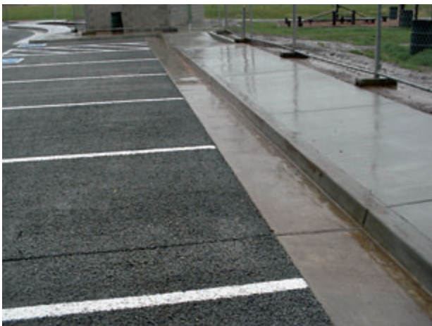
Figure 6.11. Photo of porous concrete parking area during rainy weather (courtesy of Rick Reed, Lehigh Southwest Cement).
