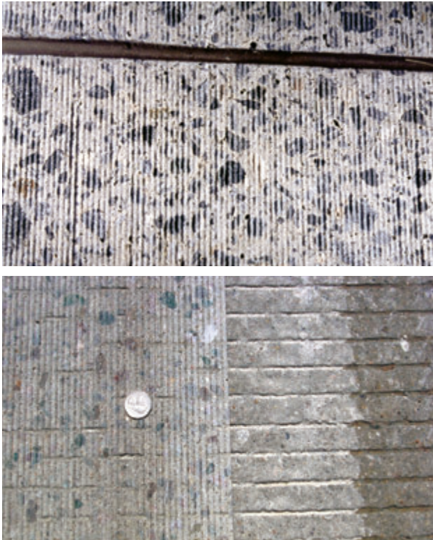
Figure 6.14. Close-up photos of diamond ground pavement (bottom photo illustrates use of diamond grinding to remove a noisy transverse tining texture). Photos courtesy of International Grooving and Grinding Association.
