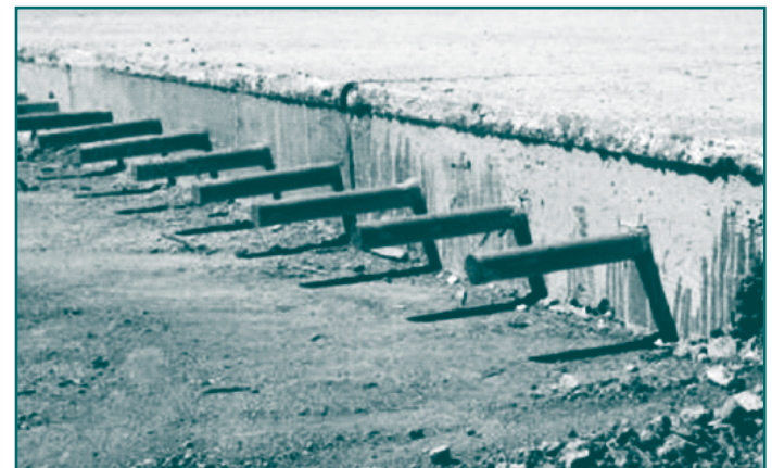
Figure 5. Photo of epoxy-coated dowel bars in full-depth concrete pavement repair (photo credit: www.pavementinteractive.org)
